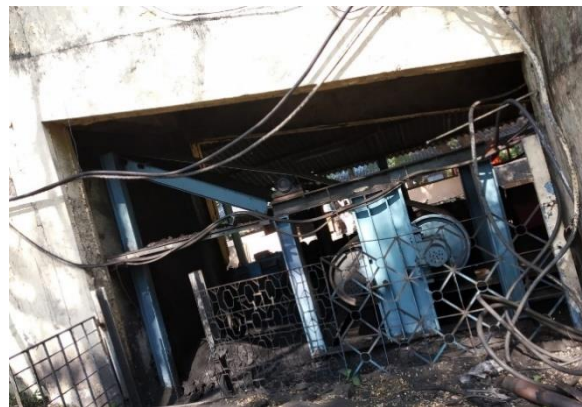
Figure 5.6 Motor drive of belt conveyor
