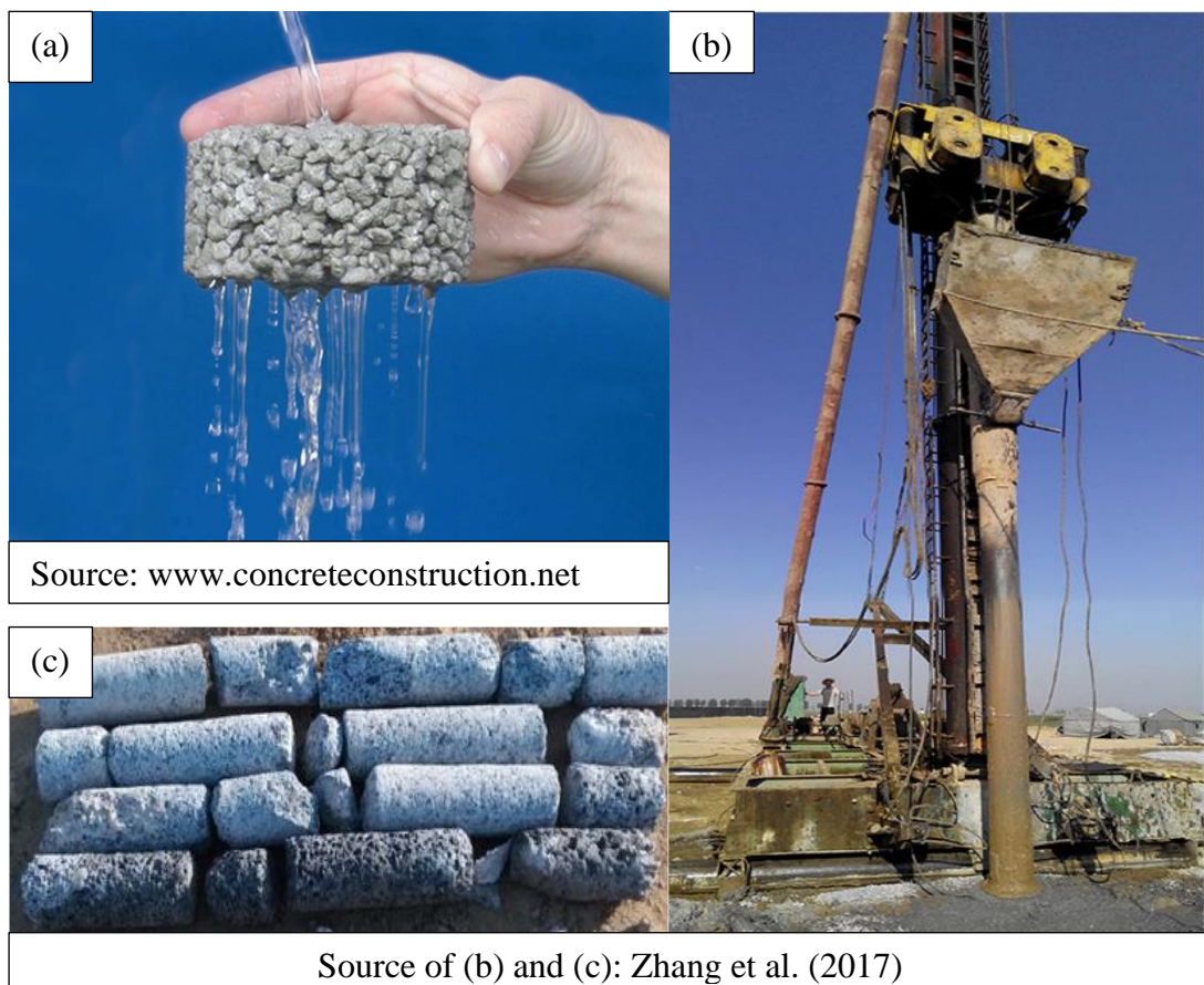
Figure 1.8 Pervious concrete (a) Sample (b) Installation of pervious concrete column (c) Core drilling samples after 28 days
