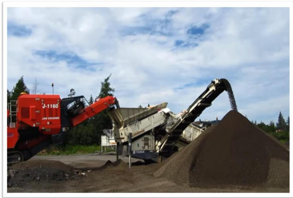
Figure 1.3 RAP stockpile at Hot Mix Asphalt Plant
