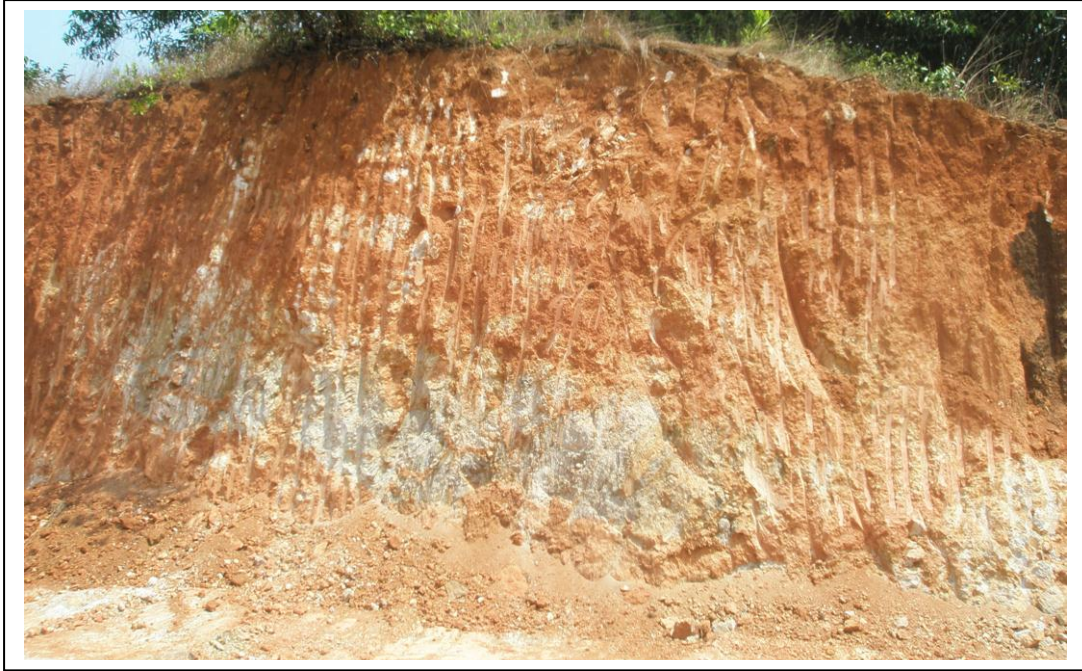
Fig. 3.17 Primary laterite (in situ) aluminous formation through spheroidal weathering of granitic gneiss at Karnire (Munkur- Inna Road)
