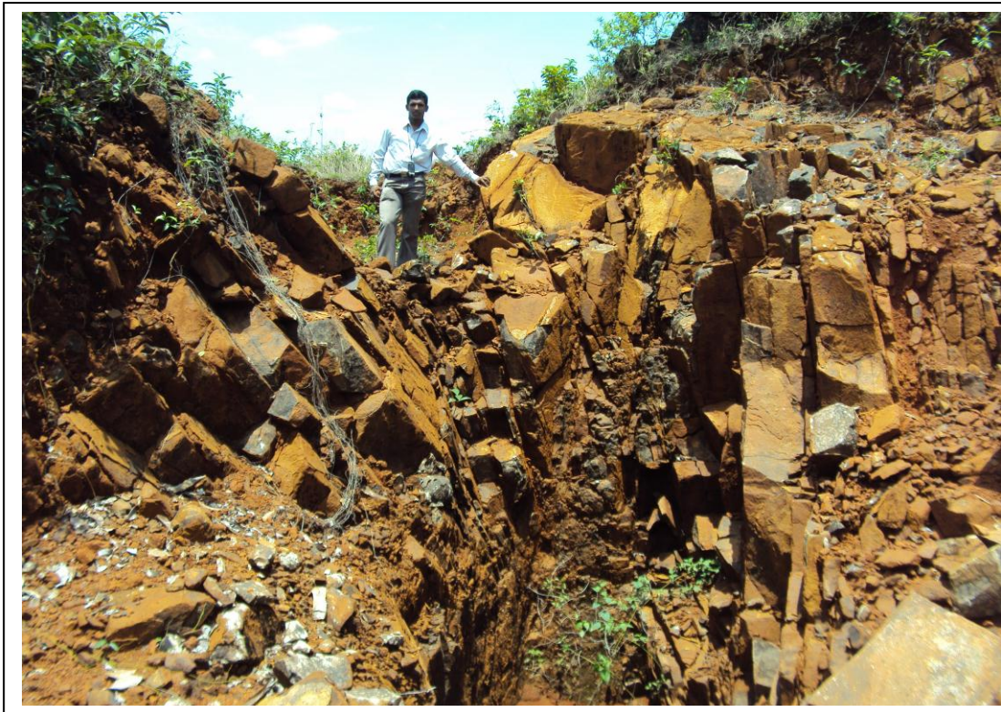
Fig. 3.14 Photograph showing the multiple sets Joints in the gabbroic mass at Bola gudde
