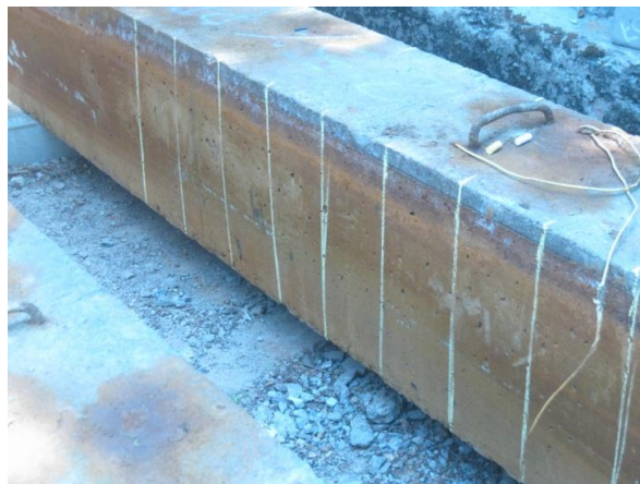
Fig. 3.6 Beam specimen marked in to number of grid to measure corrosion current density
