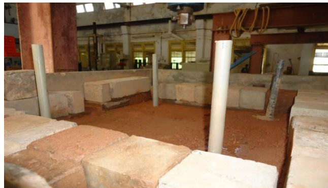
Fig 3.14. Peizometers for monitoring the level of water table
