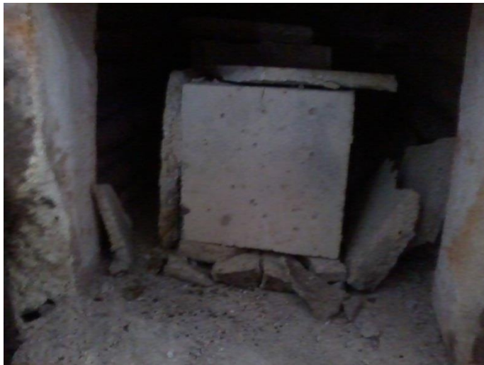
Fig. 6.1 Separation of mortar coating
