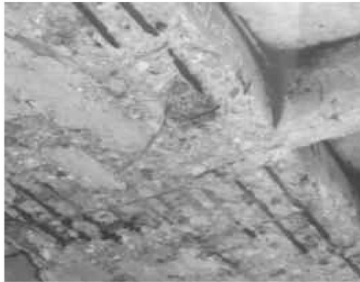
Fig. 1.1 Spalling of concrete from slab [Folic et.al. (2002)]
