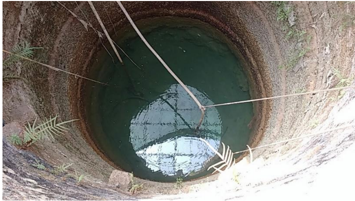
Figure 3.12 Photograph of pumping well no. 4
