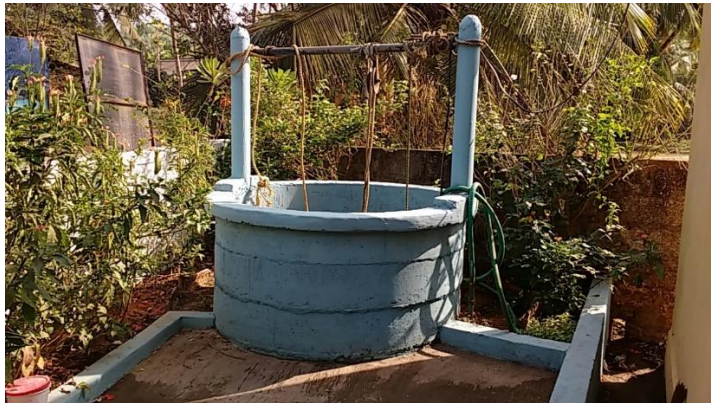
Figure 3.13 Photograph of pumping well no. 5
